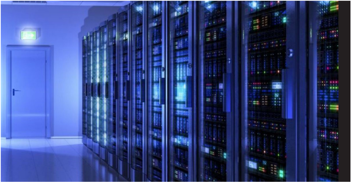
Figure 2. Image Source –Web. Data Center, 2015
